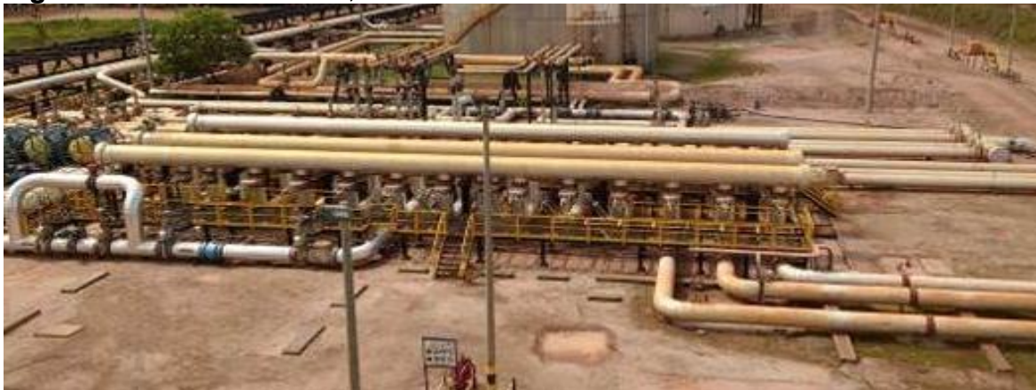
Figura 17. Manifold interno, CPF-B.
