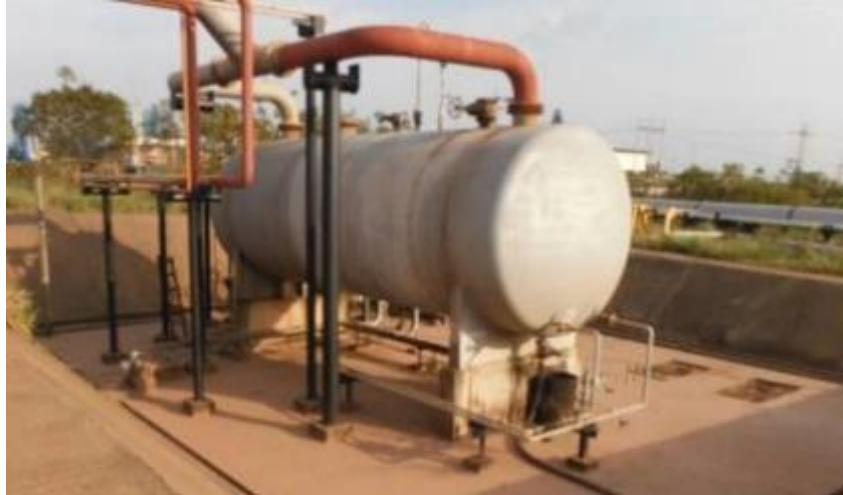
Figura 20. Tanque KO Drum, CPF-B.
